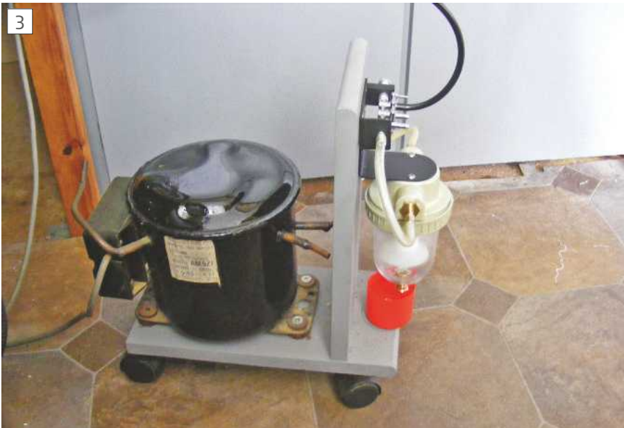
The new compressor system on its trolley.
