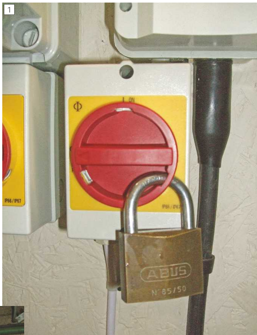
Isolator locked in the Off positioned
