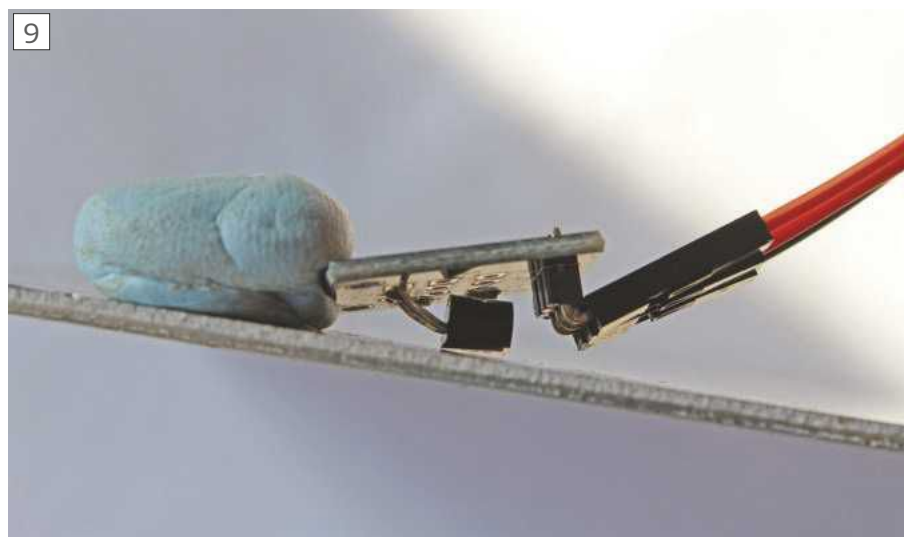
A Wrongly Placed Temperature Sensor
