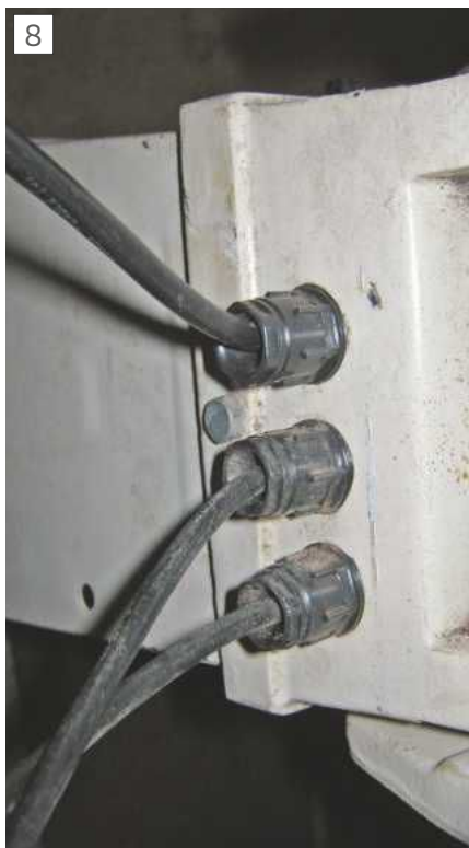
Replacement wiring gland after damage
