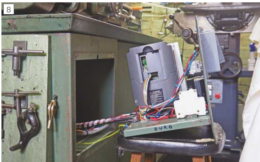
The VFD fits neatly into the space left by the electro-mechanical controls. All external controls are low voltage.
