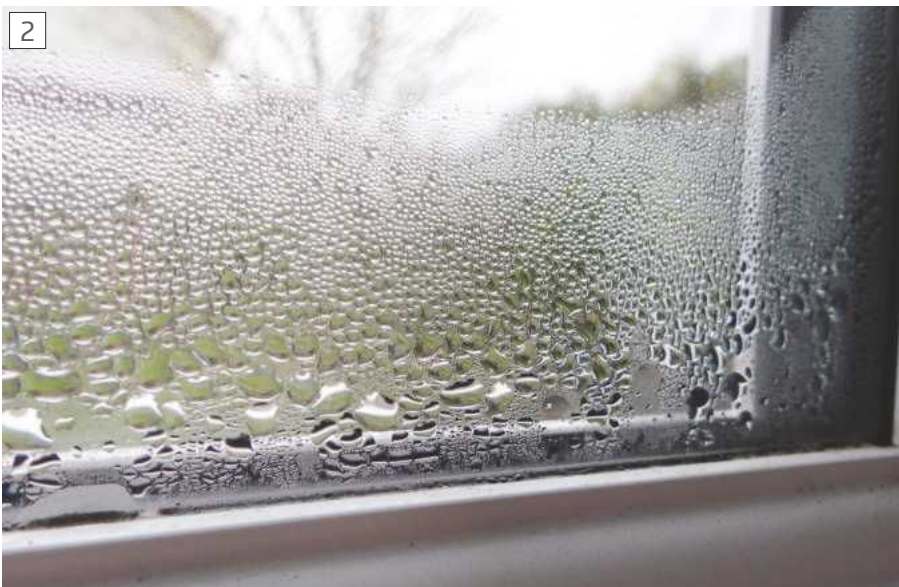
Condensation – a warning
