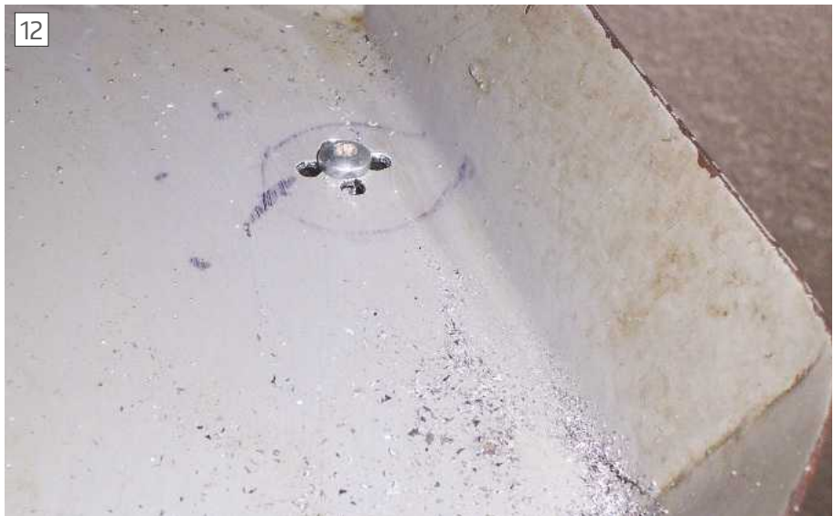
Holes in coolant tray for "new" drain
