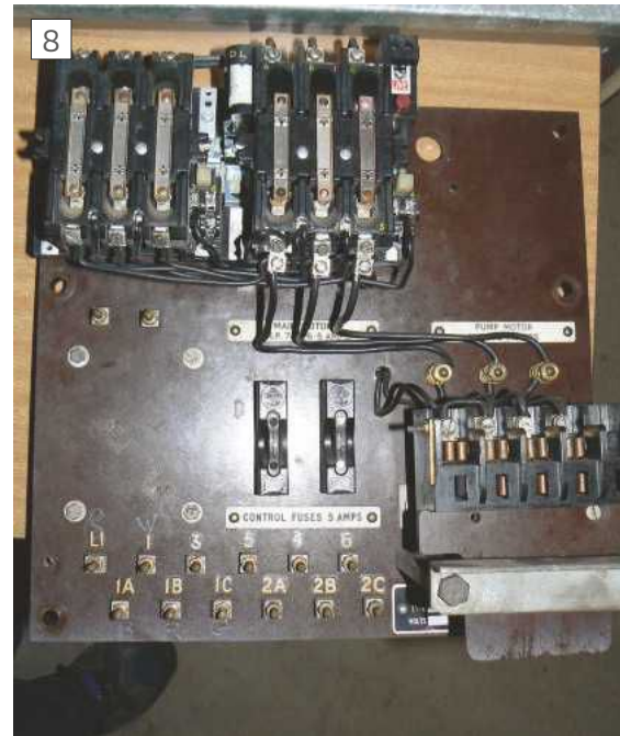
Electrical contactors on their board
