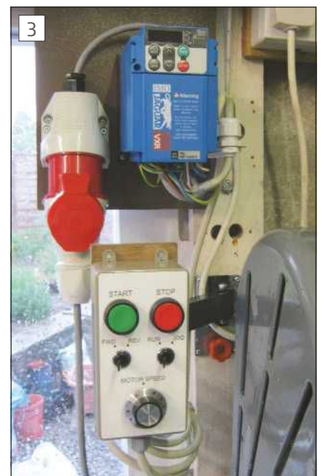
Control Panel mounted for use on the lathe
