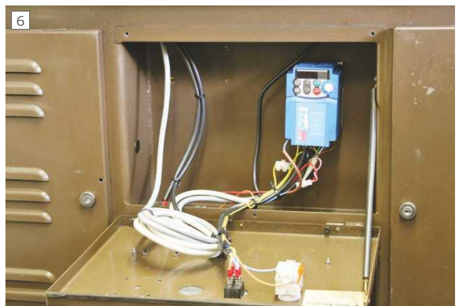
Control panel wiring & VFD (blue box)
