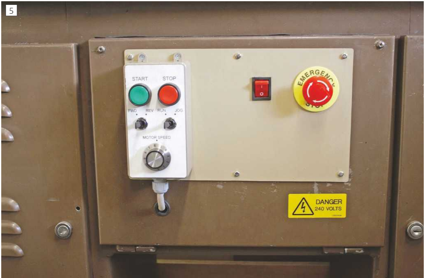
New control panel
