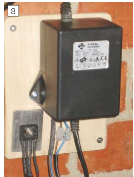
The power supply please note the wires at the bottom are 12V DC the mains supply is pre-wired and enters at the top.
