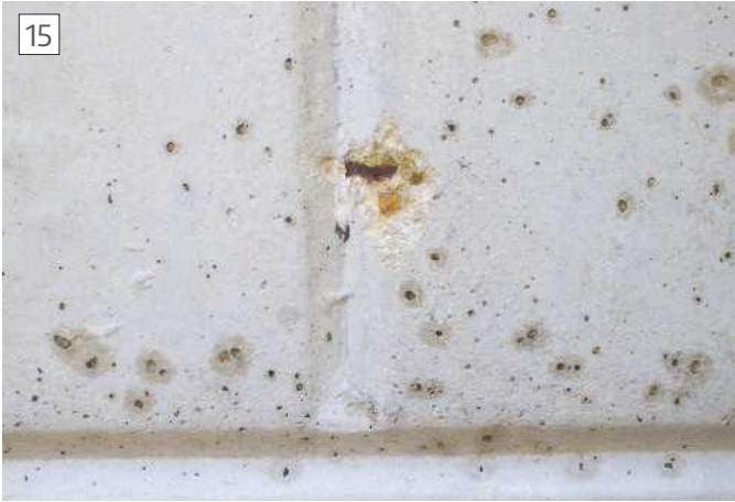
Spalled concrete and rusty re-bar
