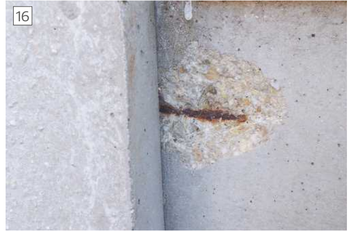
Spalled concrete and rusty re-bar
