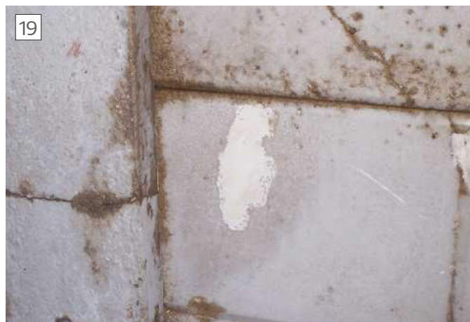
Level made good with external filler. Cracks and porous areas highlighted by silicone waterproofing solution
