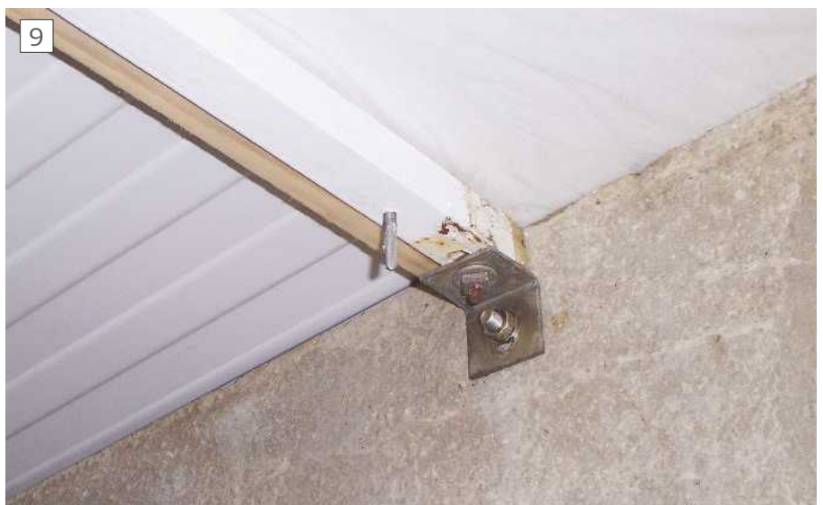
The protruding roof bolts
