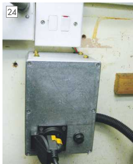
The aluminium box containing the transformer. The socket and plug are bottom left, with the fuse to the right and the master switch above the box.
