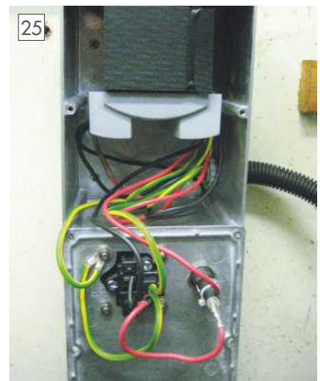
The inside of the box, showing the transformer at the top. The earth wires are also clearly seen.
