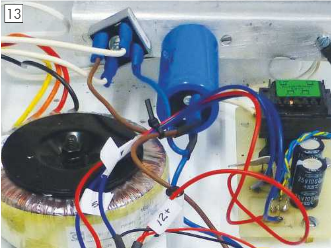
Power supply transformer rectifier and capacitor.
