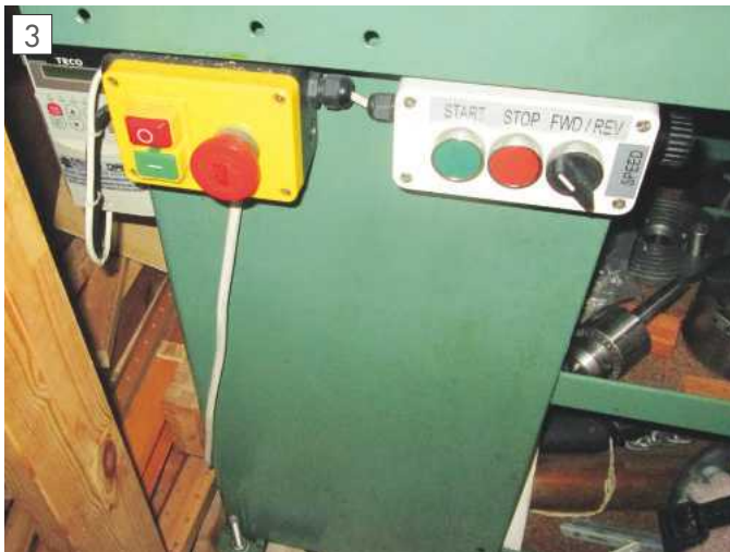
Electrical installation on Myford stand – emergency stop/NVR, inverter and remote control pod.
