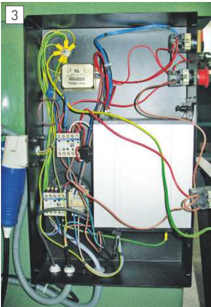
Danfoss inverter drive, zero-volt switch and associated electronics inside the black cabinet on the left side of the machine.
