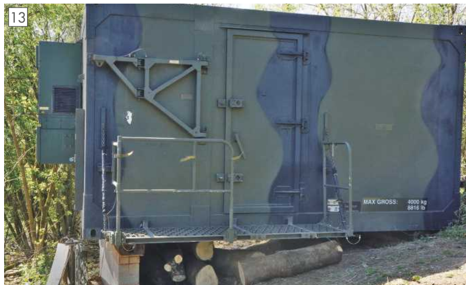
Air conditioning equipment.
