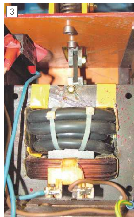
The new secondary winding.
