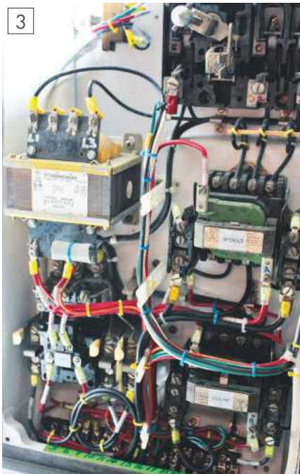
The mill's rather complex control gear.
