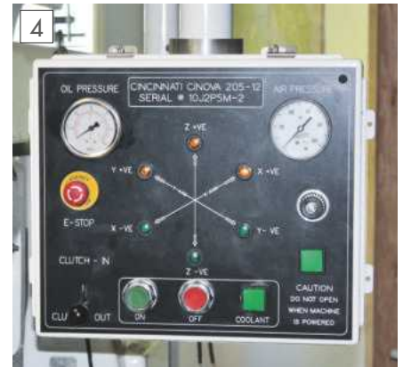
The new control panel.
