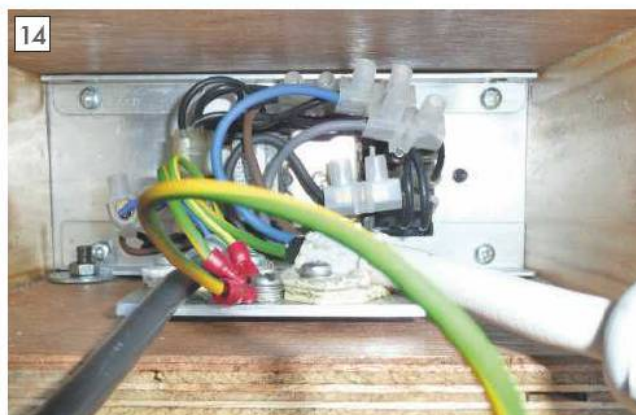
Control switch assembly in plinth.
