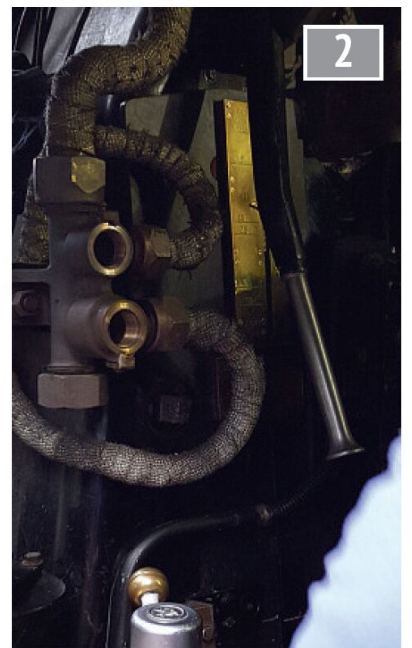
Where the reverser plate gauge is mounted.
