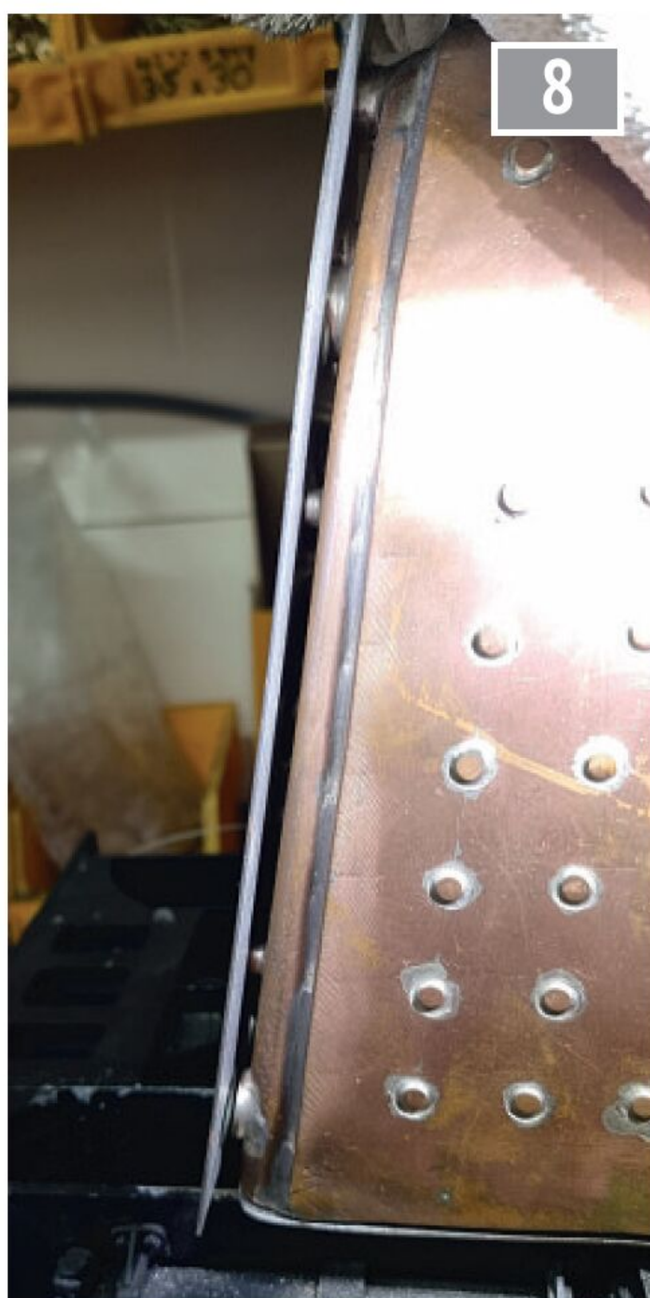
Clearance between the cleading and the boiler.
