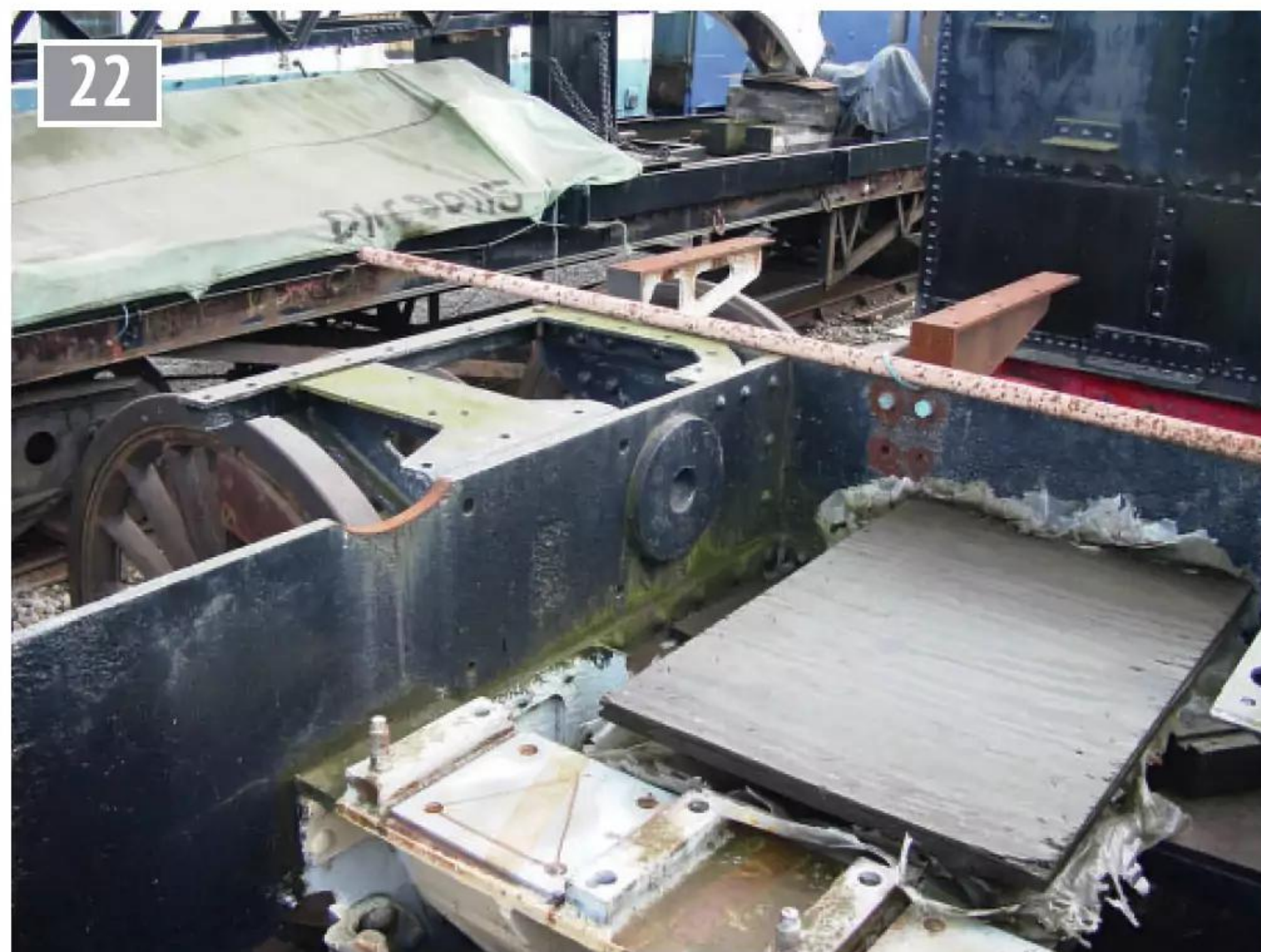
One of the boiler mounting pads on the drag box.
