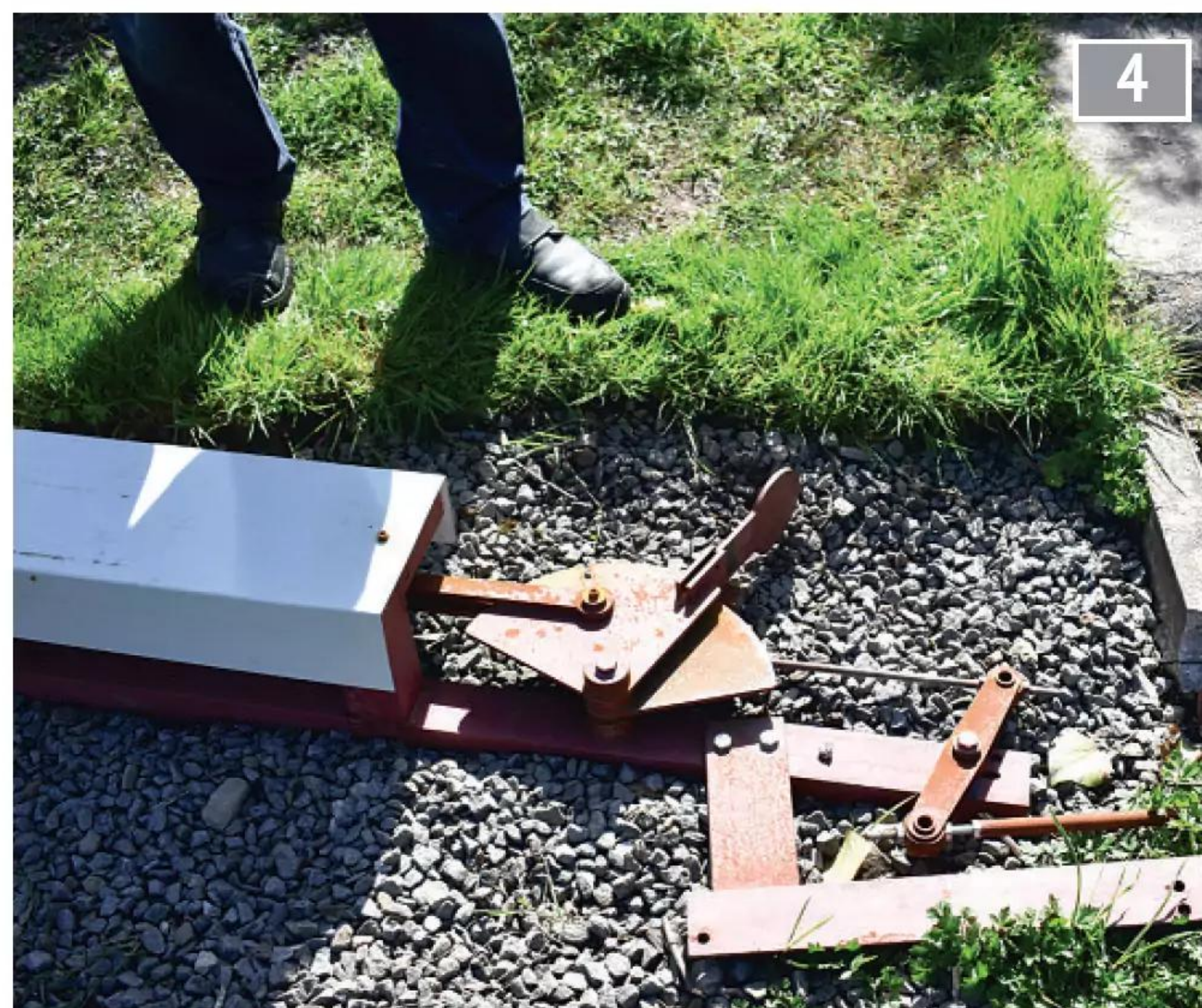
The motor attachment to the point mechanism with the indicator plate horizontal showing it is being manually operated.
