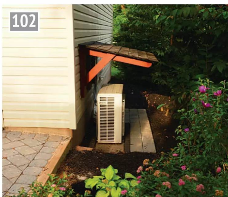
102 The outdoor portion of the Mini Split heat pump system, sitting on its pad on the north side of the shed. The roof above prevents wintertime snow from burying the heat exchanger and hampering its operation.
