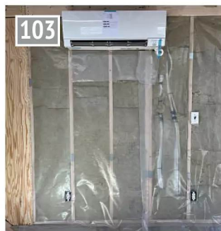
The downstairs indoor heat exchanger, silently blowing nicely warmed air around the newly insulated and vapour-barriered workshop in February.
