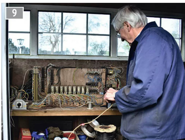
Don Burrow working in the signal box which controls all the working signals on the track.
