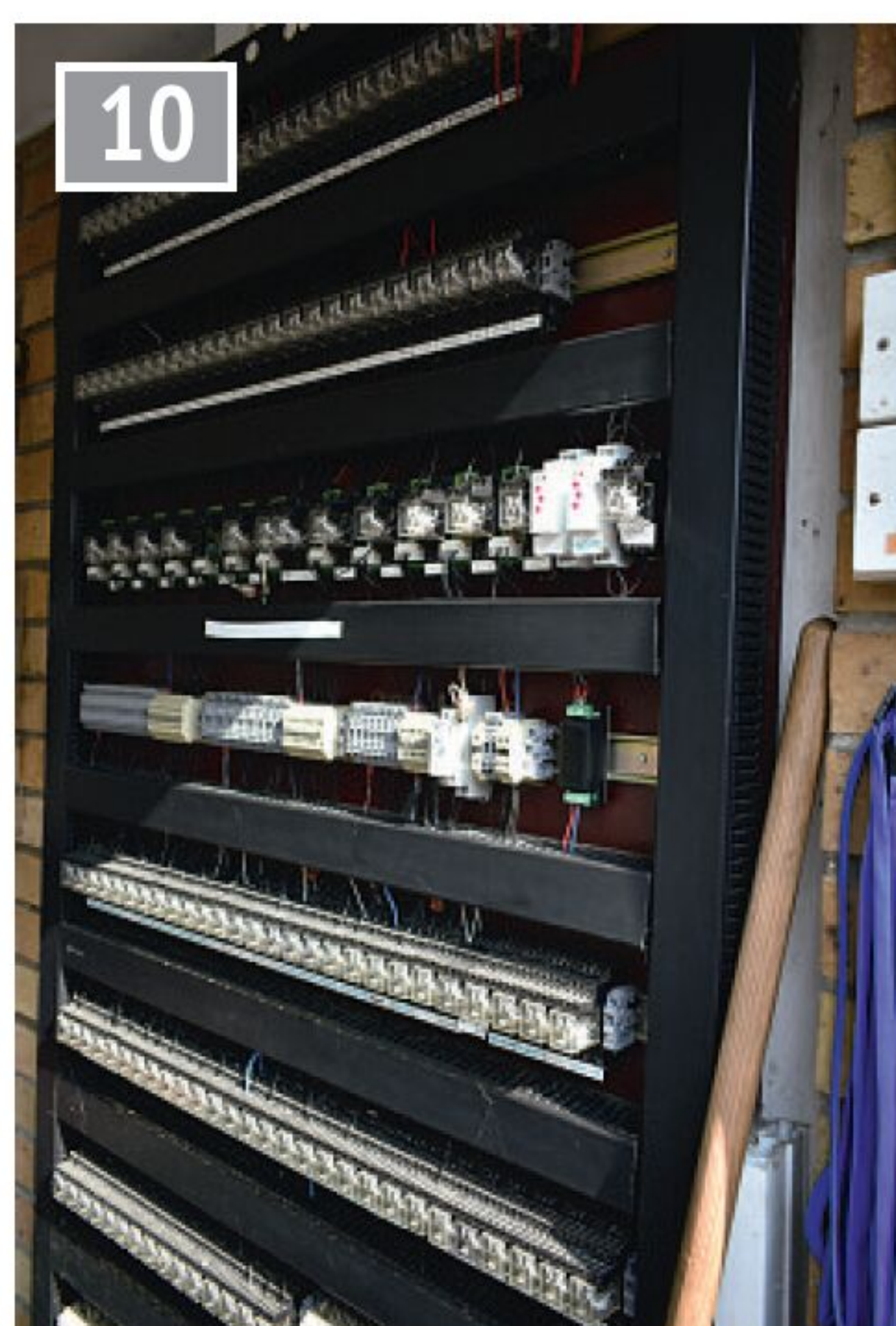
An impressive relay board in the signal box.
