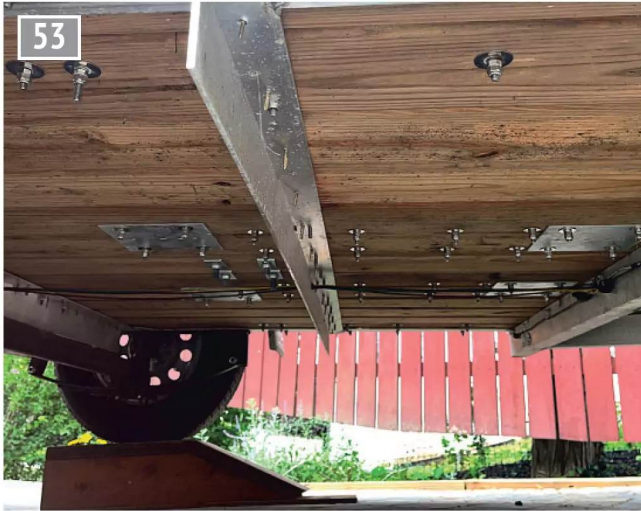
53 A hundred (or so) quarter-inch diameter stainless steel fasteners, all lock-nutted to be sure, secure the E-Track strips to the trailer's floor and chassis. A chain is only as strong as its weakest link, after all.
