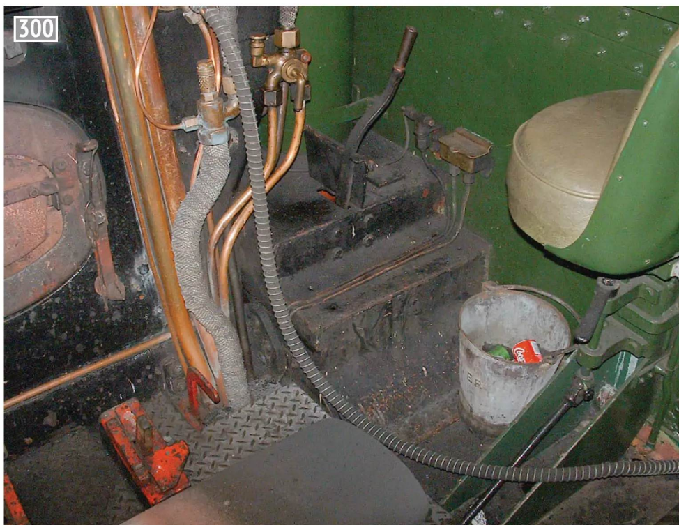
Right-hand water valve – lever below seat (photo by John Thompson).
