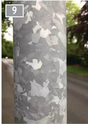
A zinc-galvanised steel lamppost – a common sight on many streets. The crystalline structure of the zinc plating can clearly be seen.
