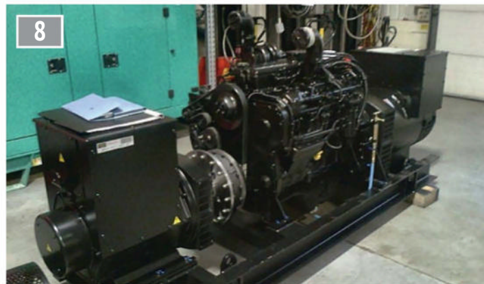
8 The Cummins diesel engine was chosen and installed. Photo David Moore, 2012.
