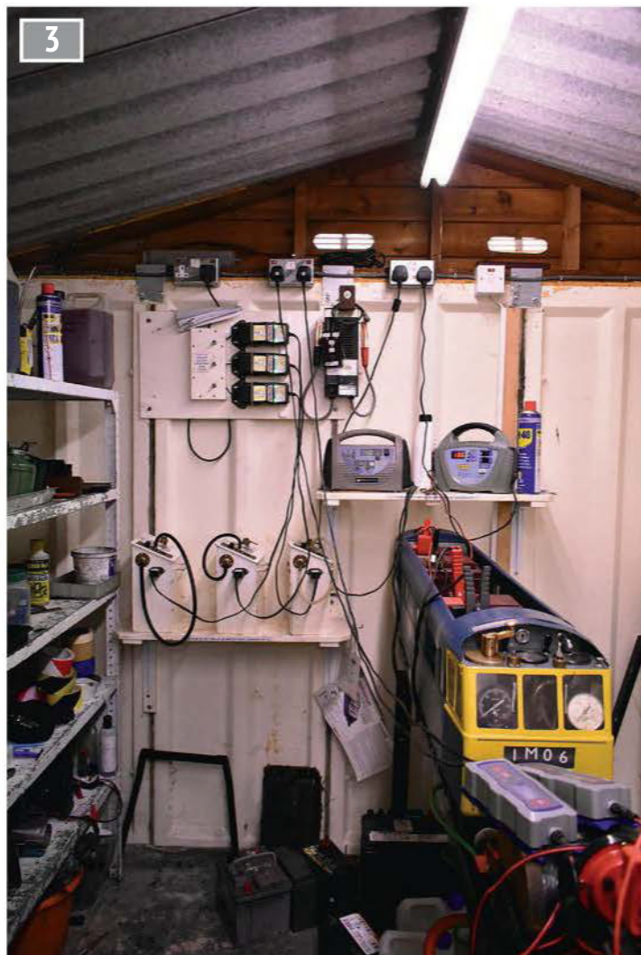
The battery charging points in the locomotive shed.
