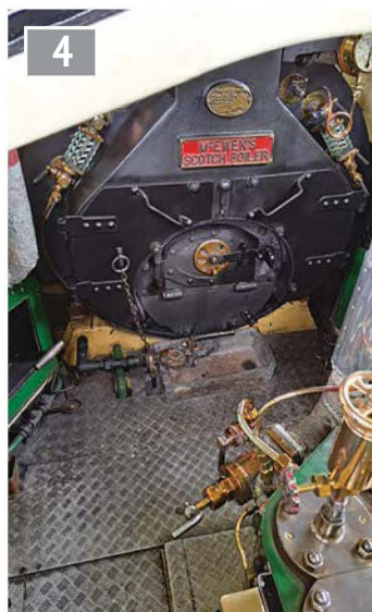
SL Nuneham boiler.
