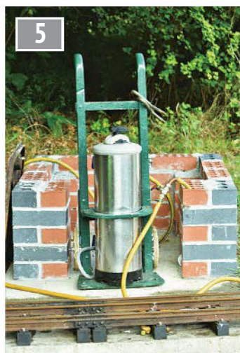
The portable water softening plant for the track.
