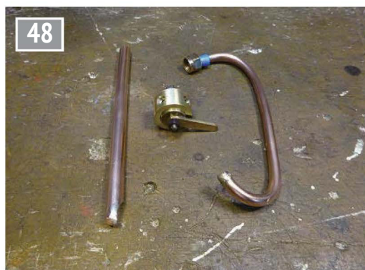
Reversing valve cleaned.
