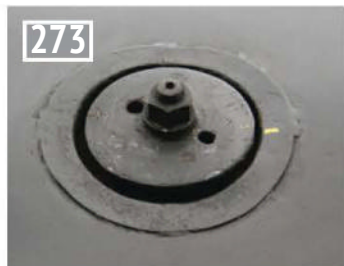
A close view of a washout plug.
