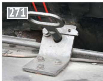
Blow down valve operating handle.
