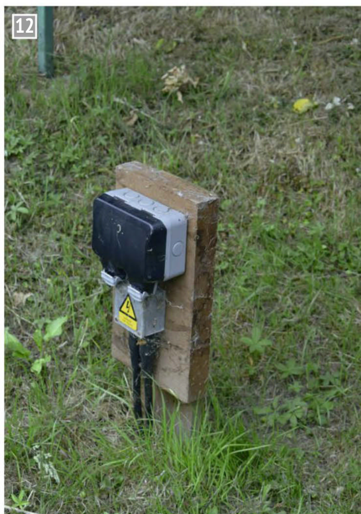
A useful mains power socket; just one of many dotted about the site.
