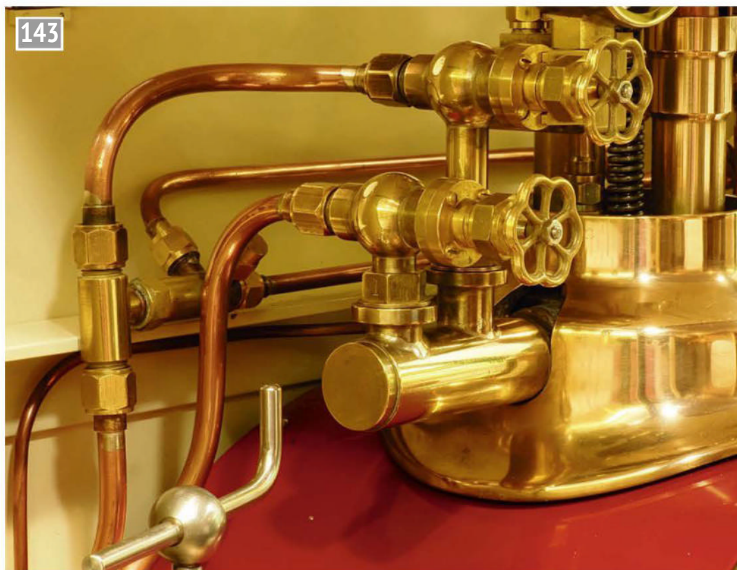
To the left, the vacuum ejector is to the D.A.G. Brown design. The tee behind the ejector contains a check valve to prevent the vacuum system being pressurized should the exhaust become blocked.
