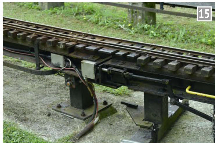
A good solid traverser lock and operating mechanism.
