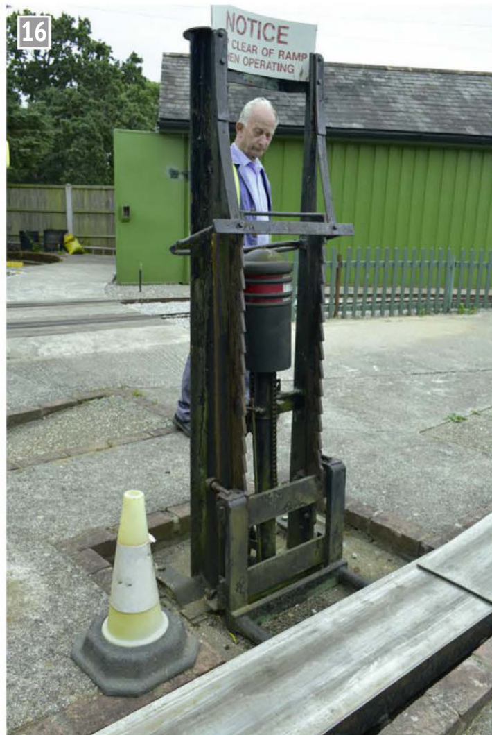
The heavy duty hydraulic lifting point at the steaming bays.
