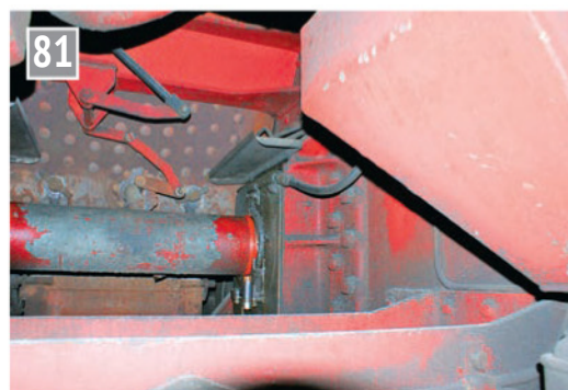
Linkage to the blowdown valve.
