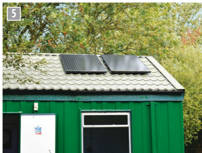
Solar Panels on the clubhouse roof.
