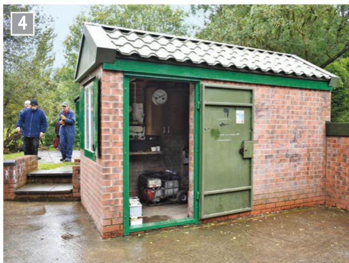
Traverser operating shed with compressor and battery storage.
