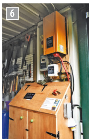
Control gear and inverter for the solar panels.
