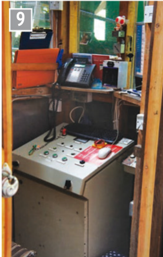
9 Control cabin at top station. Normally three staff are on duty.
