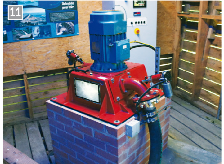
11 CAT water turbine generating about 3.5kW fed by water from the reservoir above.
