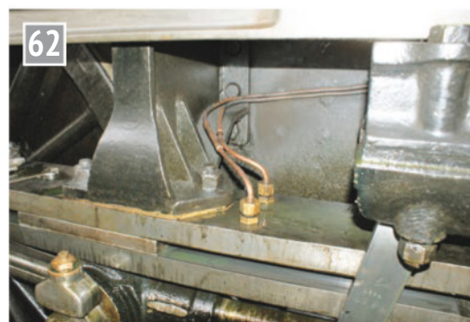
Lower end of the support bracket – note packing.
