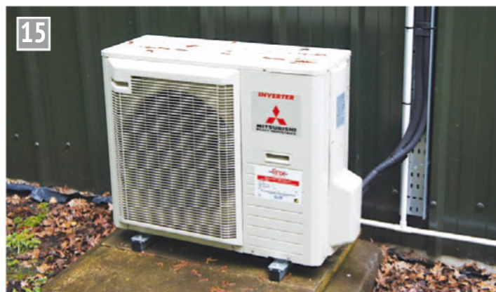
The Mitsubishi air source heat pump has so far proved very effective at heating a large space.
