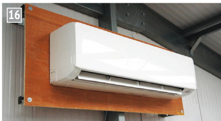
Mitsubishi air source heat pump outlet inside.
