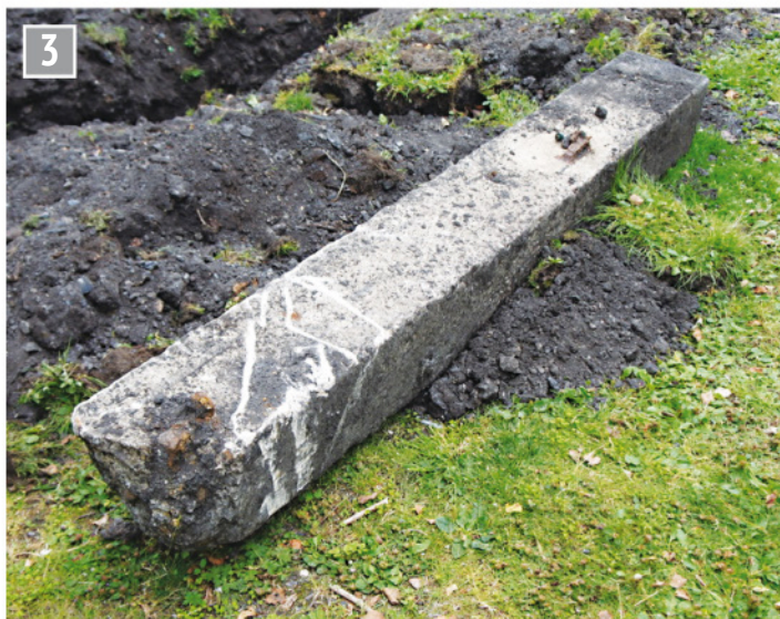
Old gatepost found during excavations, one of several obstructions to construction and electric supply installation.
