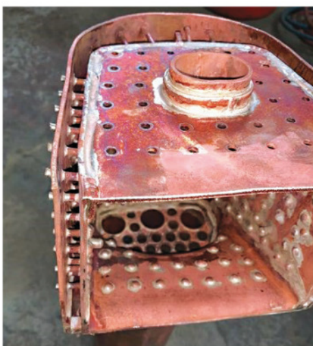
7. These pictures show the stay and firehole door penetration, all looking excellent.
