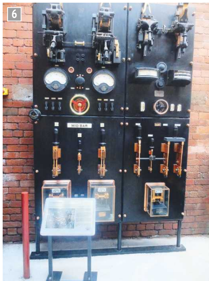
Switchboard at Bolton Steam Museum.
