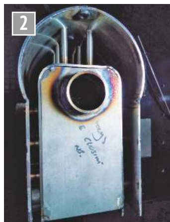
Inside a larger boiler designed to the Australian code.
