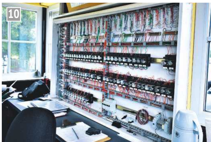
The impressive relay panel in the new signal box.
