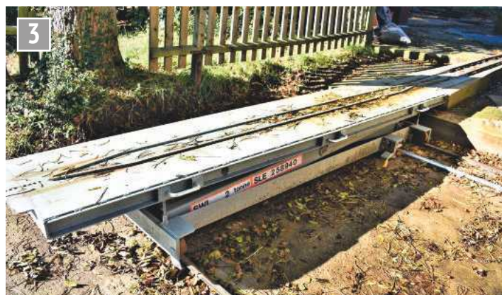
The newly installed 2 ton Hydraulic lifting table.
