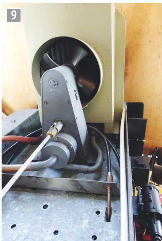
The water pump.
