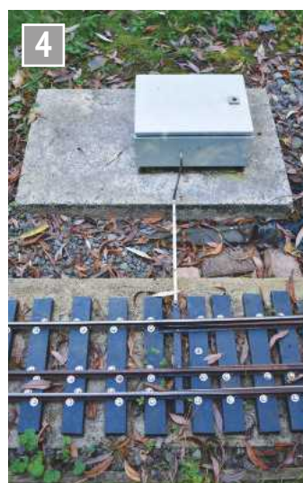
One of the simple point control boxes showing the new plastic sleepers.
