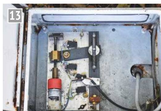
Inside one of the point motor control boxes showing the micro switches for blade detection.
