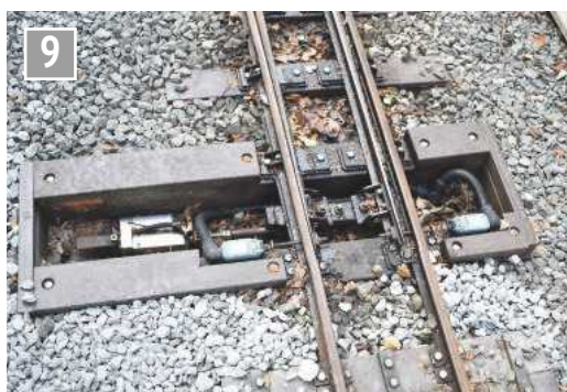
One of the compact point operating mechanisms complete with blade contact sensors.
