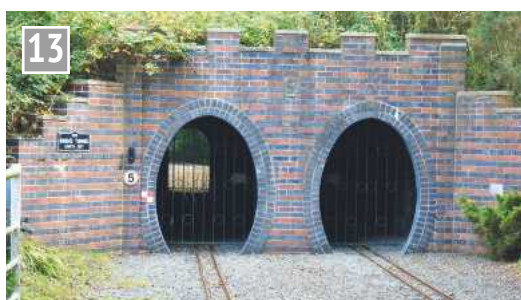
The twin bore Wren Tunnel.
