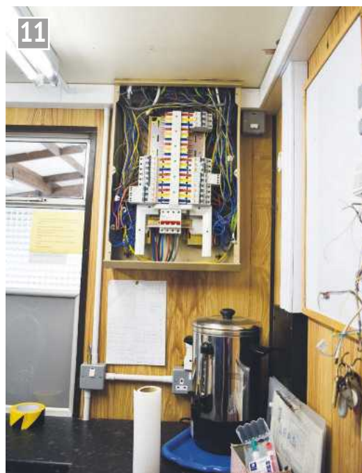
The new power installation box and distribution board at the station.
