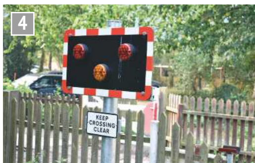
Flashing lights display on the main road crossing.
