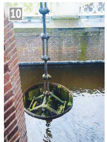
Pump set in the collar launder. Beams lift the bucket pumps with their D-shaped clack valves raising water to canal level.
