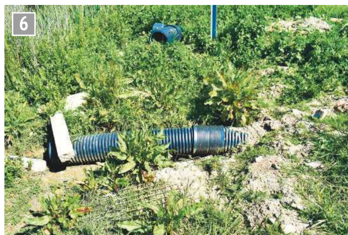
The land end of the new cross site drainage pipe needs another connection chamber.
