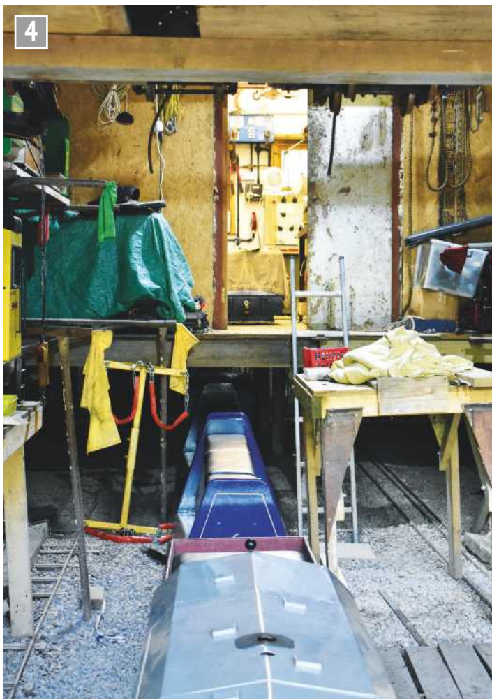
The view inside the carriage shed showing the main workshop floor level which was also flooded.
