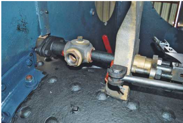
A close up of the take-off from the rear main steam pipe for the left-hand injector steam feed.
