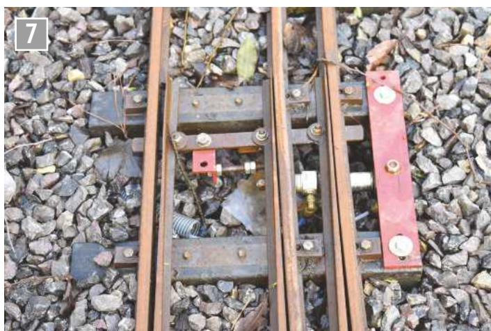
One of the new pneumatic point operating installations.
