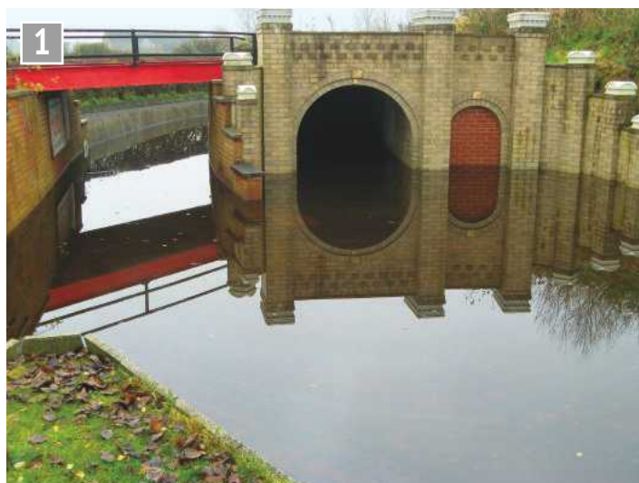
The flooded tunnel at SFMR. (Photo courtesy of Barbara Smith.)
