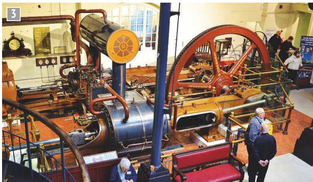
An exception to the norm: pumping against a head of water, the horizontal cross compound engine at Kew, from Waddon Pumping Station near Croydon, unusually required no governor to stop it 'running away' during its working life.
