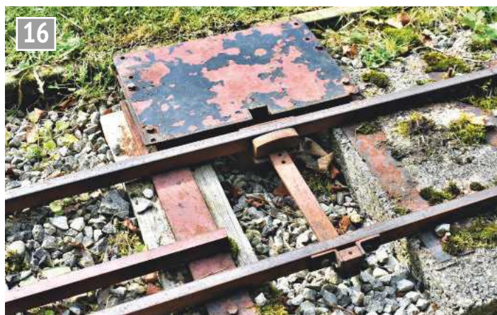
One of the track circuit 'flip flop' switches.
