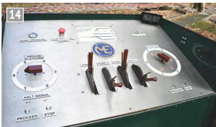
The comprehensive yet well planned control cabinet on the ground level track.
