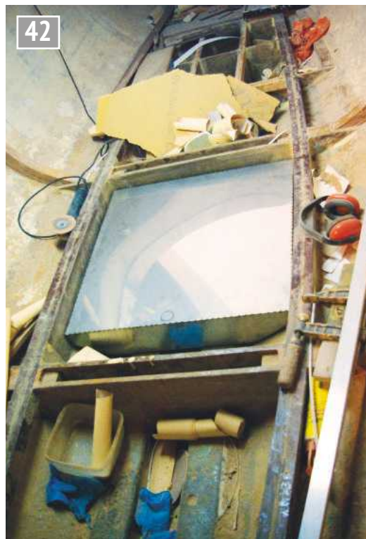
A tank for water under the boiler.
