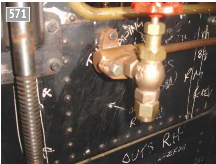
Injector steam valve.
