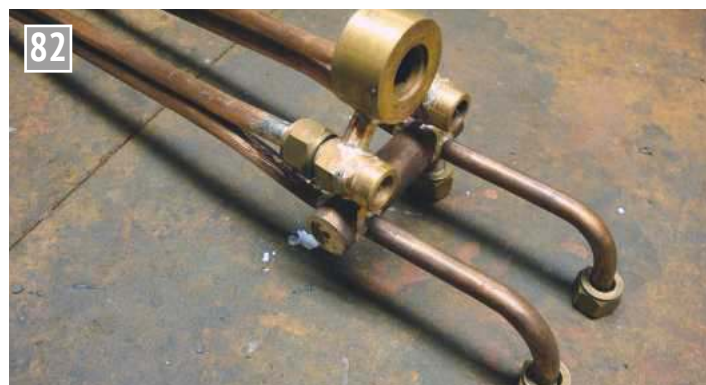
82 Reconfigured superheater; it can be installed and removed through the smokebox door – but it is necessary to remove the chimney and top of the smokebox to get at the nuts. See also photo 84.
