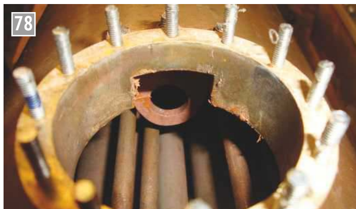
View through dome bush with regulator removed showing bracket installed to support main steam pipe. Note how the longitudinal stays are anything but straight. Testing at 160 psi made no detectable difference.
