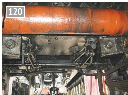
Drain cocks under the cylinder block.
