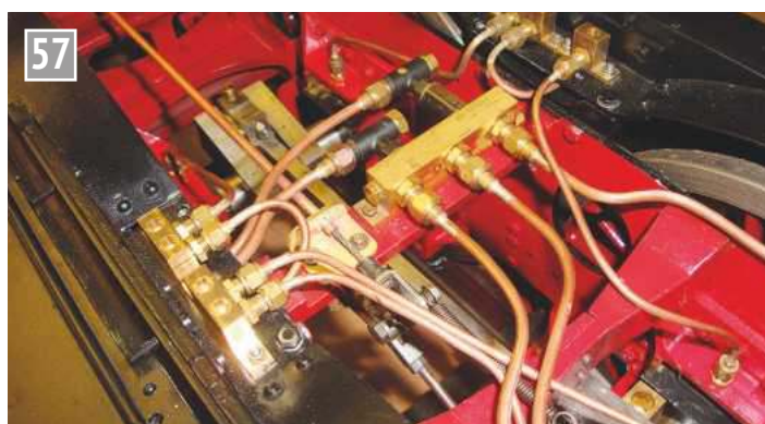
57 No 4497: In the middle of the photo can be seen the crank where the mechanical drain cock linkage changes to a Bowden cable. The springs return the drain cocks to the 'closed' position. Also in the picture can be seen the manifold where the single feeds from the two mechanical lubricators split into three feeds, one for each cylinder. Oil feeds to hornblocks, inside cylinder slide bars, and weighshaft bearings are accessed through the hatches in the streamlined casing.
